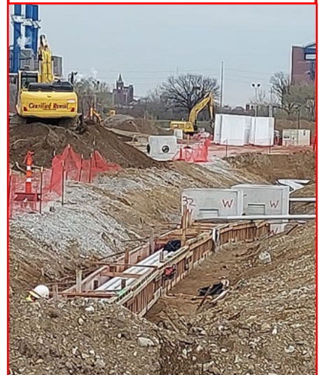
Electrical duct banks
