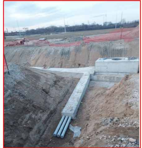
Electrical duct banks
